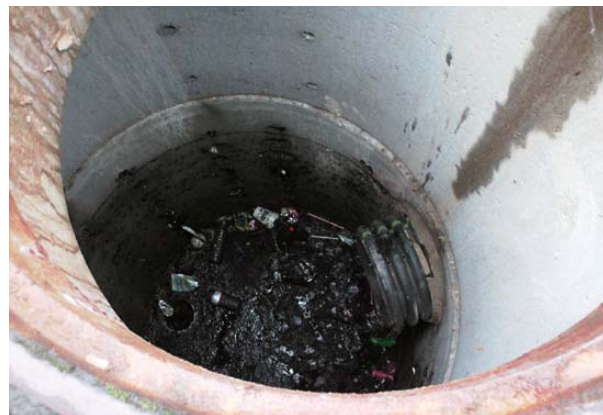
▼ PROBLEM: Trash has collected inside the drywell.
