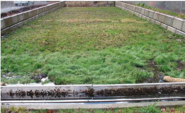
GOOD: A biofiltration swale showing a sediment trap in the foreground.
