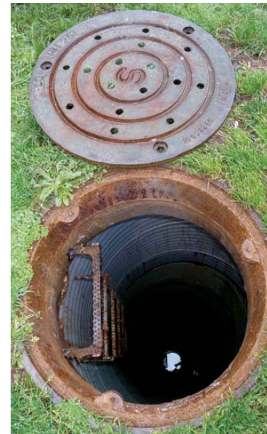
GOOD: Lid and entrance to an underground detention facility.
