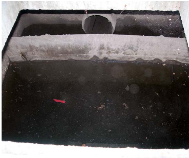
GOOD: A well maintained “API type” oil/water separator.
