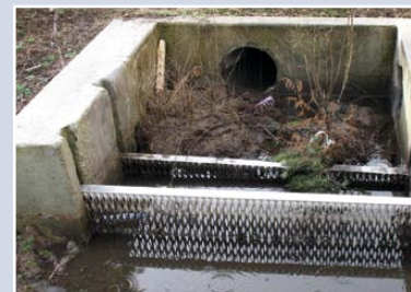
▲ PROBLEM: This trap needs cleaning.
